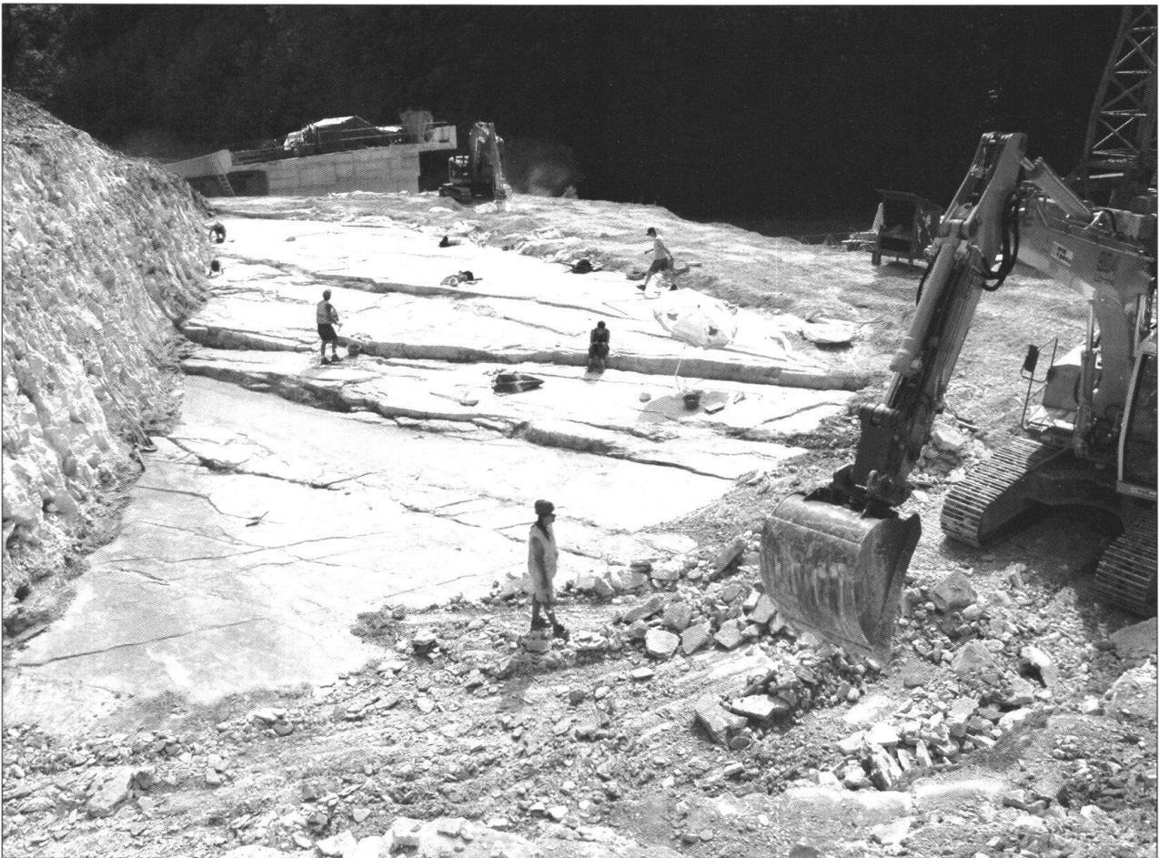
Fig. 3: Excavation of the main track level at the Chevez - Combe Ronde tracksite. This site is protected by the extension of the highway bridge, which is visible in the upper left corner of the picture.
