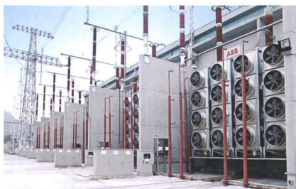
HVDC-Installation in China.
