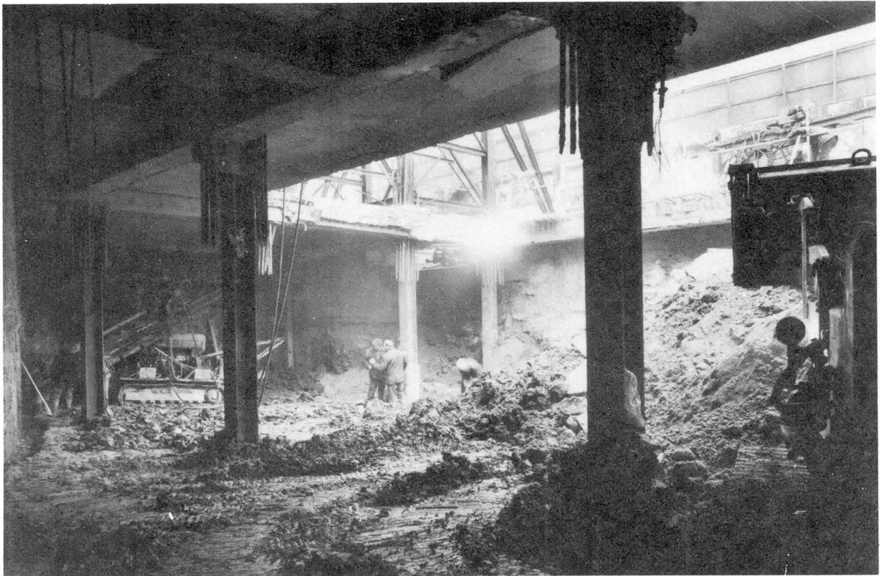
Fig 1 Ground anchor installation and excavation beneath the ground floor slab of a basement substructure, Victoria Street, London
