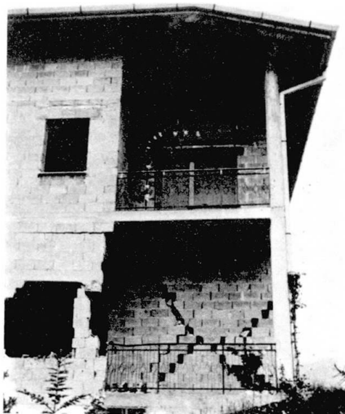
Figure 13: Dwelling house with workshop near Artegna. Basement in reinforced concrete and the upper stories in masonry without framing. Typical diagonal cross cracks in a wall of the ground floor.
