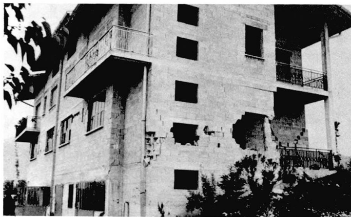
Figure 5: (after May 6th): Residential building with workshop near Artegna with a reinforced concrete cellar and two floors in concrete blocks. The side walls by the entrance incurred gaping X-shaped diagonal cracks due to the high shear stress. These cracks led to partial collapse of the masonry. The highly strained window jambs on the longitudinal façade were badly cracked.
