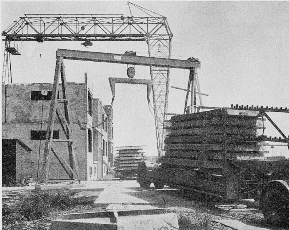
Fig. 4.2 - The Rottinghuis-housing system. The lorries with the floor elements are unloaded from the trailer by a fixed crane. In the background the portal framed crane for mounting the elements.
