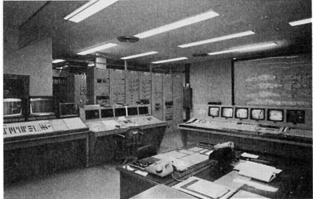
Photo 5 Control center for station building
