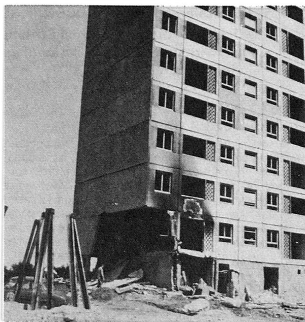
Large panel building in Algeria, Granström & Carlsson (1974). An explosion in the ground floor caused considerable damage in the panel structure without damaging the elements above.
