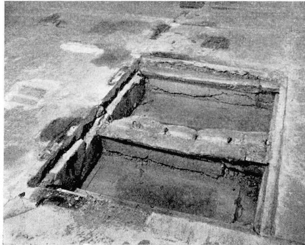
Fig. 7. Box-Section Bridge — Loading No. 7 — Shear Failure in Webs of Beams and Diaphragms.
