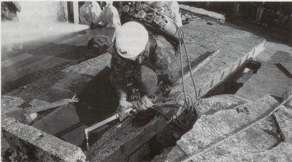
PHOTOS: RMINFO, PULLY
