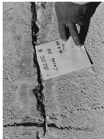
Figure 8. Crack to be sealed before injection.
