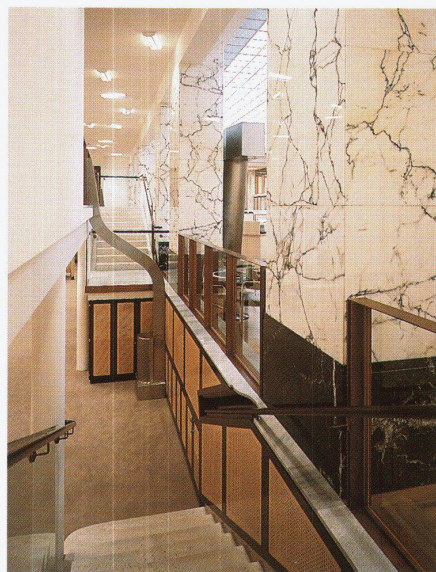
■ Gallery to one side of the main hall. Fresh air blowers with wide-angle nozzles and one of the air supply systems in the new intermediate floor.
