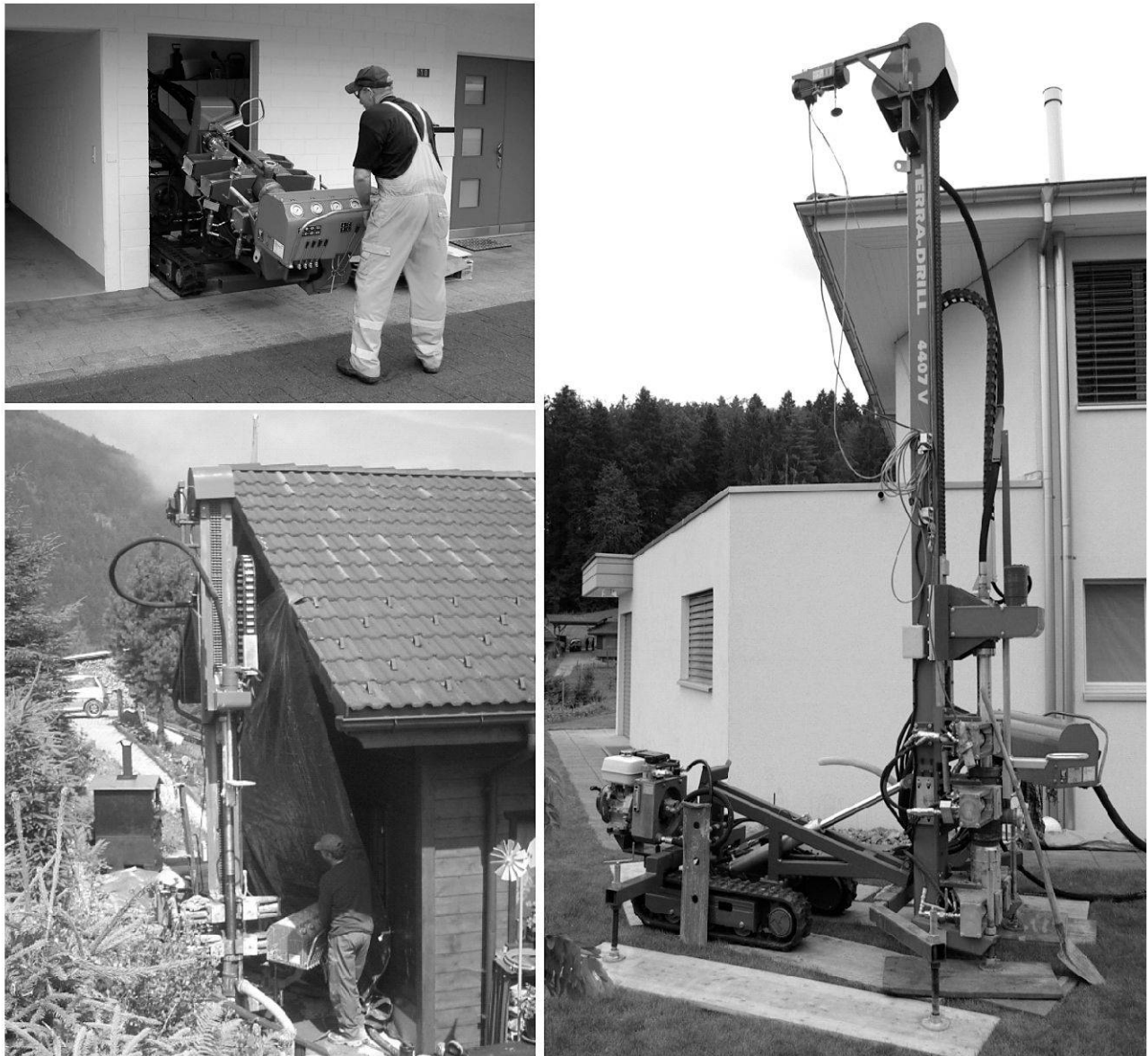
Fig. 5: Light and compact mini-rig to drill shallow [100–120 m deep] wells for deployment of geothermal heat pumps systems [source: Terra AG and J. Wettstein].
