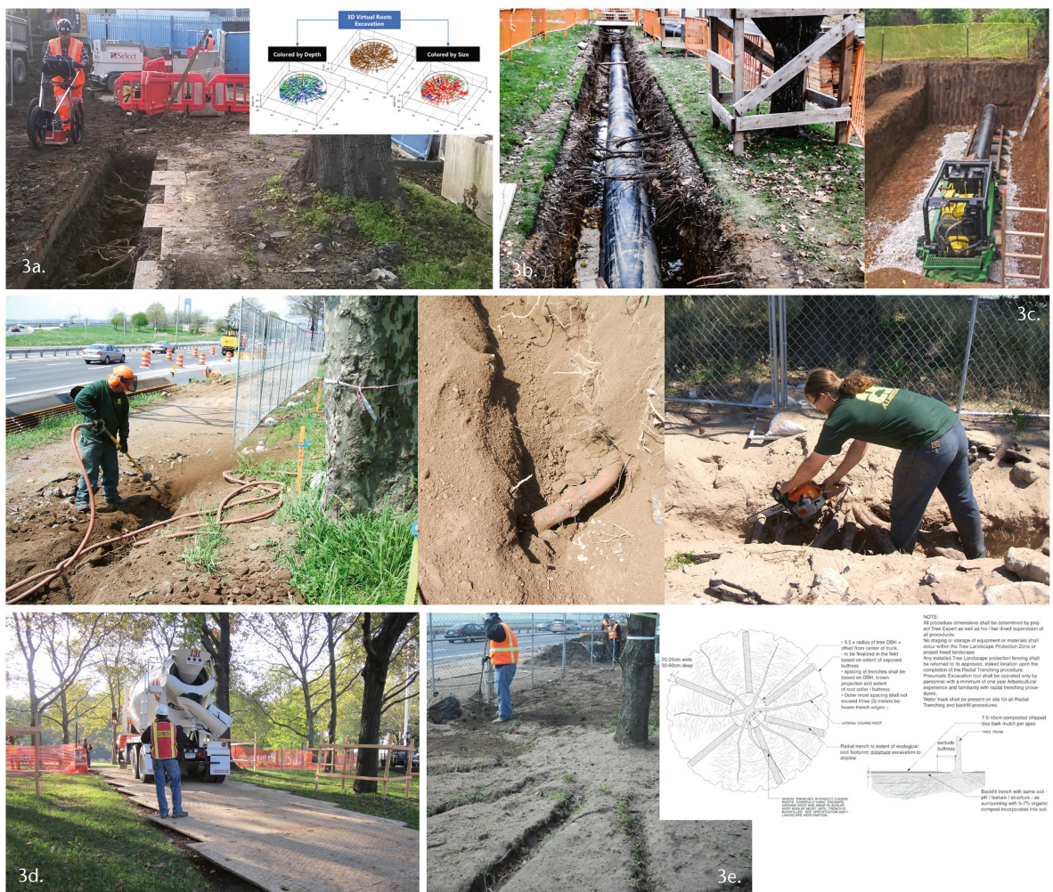
Fig. 3 Building WITH Trees®: a) tree radar GPR mapping; b) design – trenchless technology; c) pre-construction – pneumatic excavation + root pruning + tree protection zone fencing; d) ground protection mats over mulch; e) radial trenching and detail. Credits: Carsten Glaeser, Naomi Zürcher, Tree Radar
