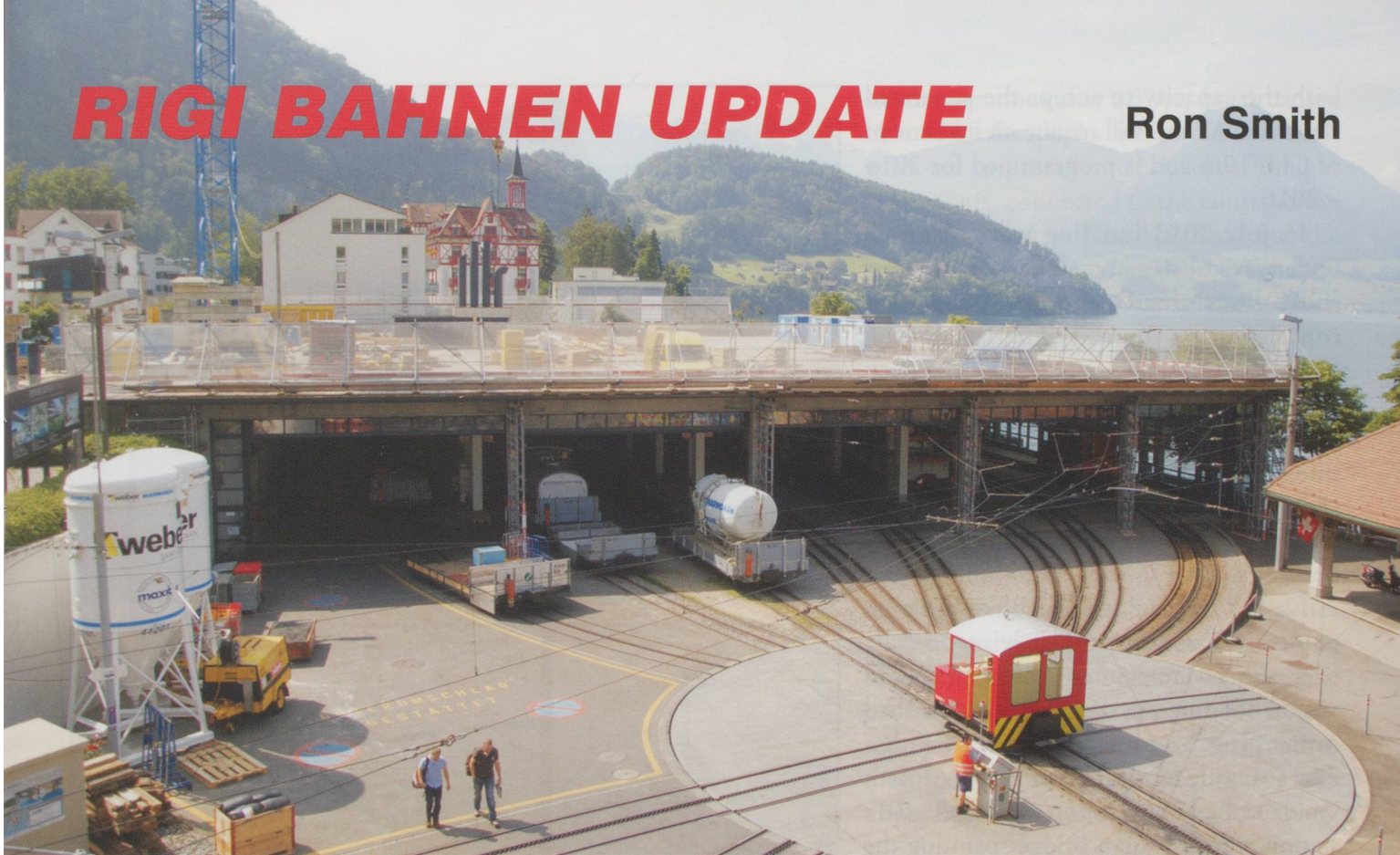
Building work on the shed roof as Ta 2/2 no 1 shunts cement silos Vitznau.
