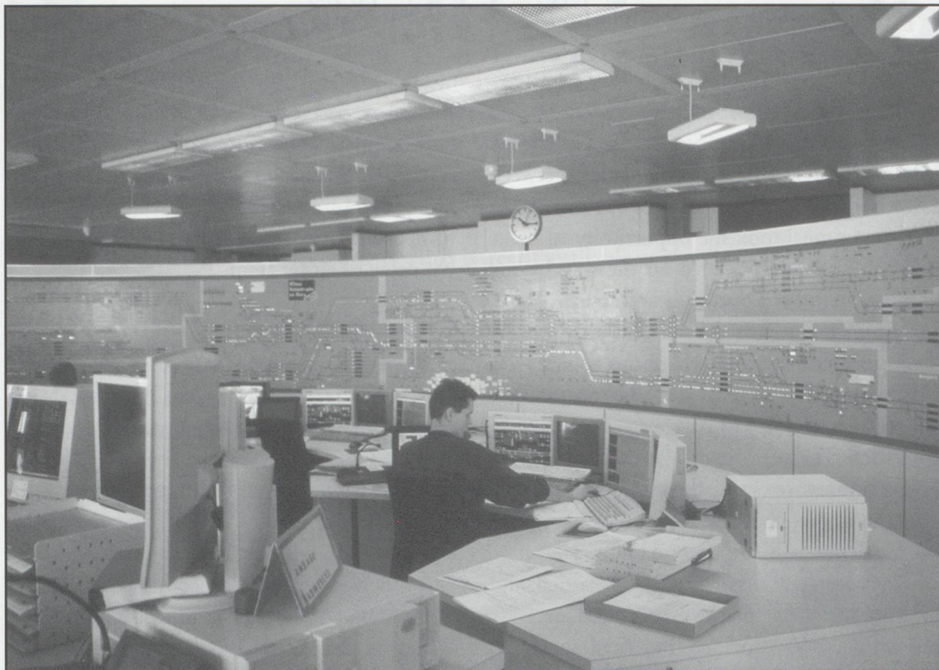
Olten Control Centre mains panel. The ETCS section is worked on a separate VDU (IECC) type panel.
