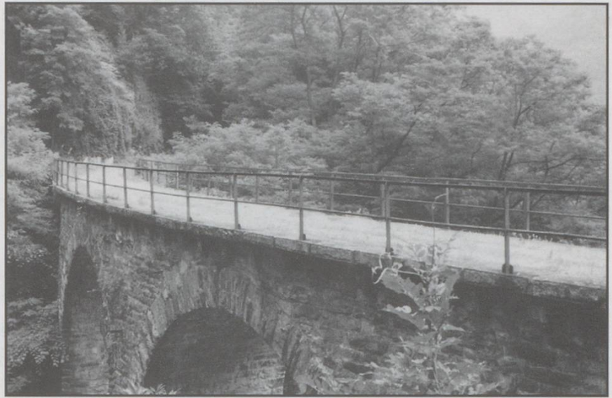
From Mesocco to Soazza the line winds along the mountainside through thick woods. This bridge spans a stream, viewed towards Mesocco. The handrails, although rusted, are still sound.
