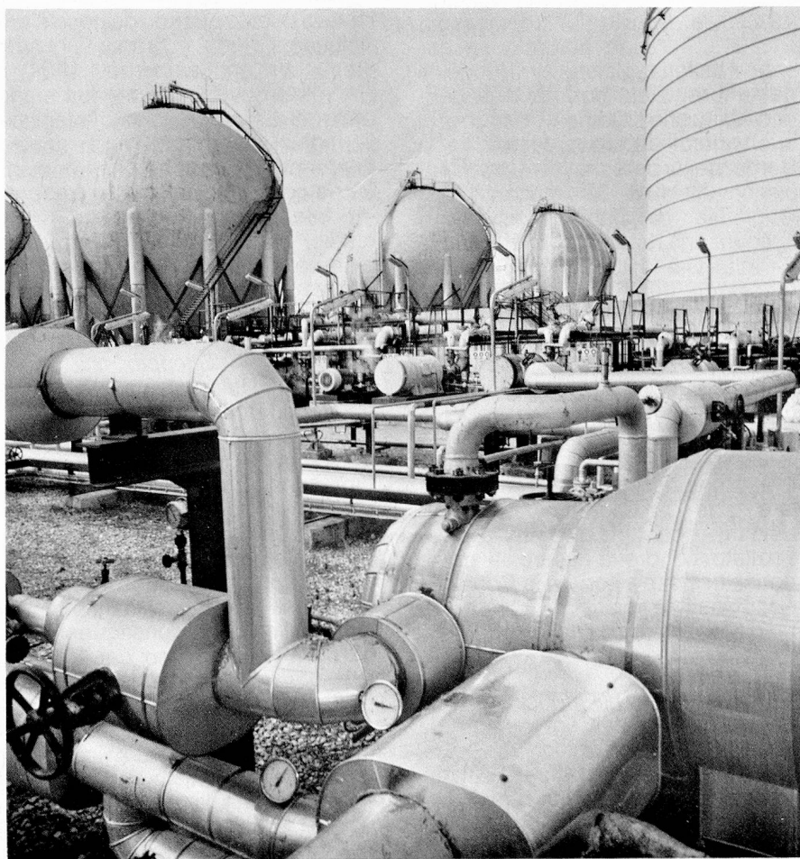
Storage facility with spherical tanks for petroleum gases, with refrigerant evaporators in the foreground.
