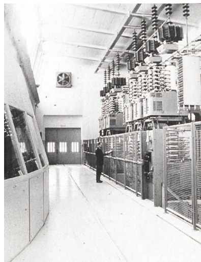
Kontrollraum in Gotland (1954).
