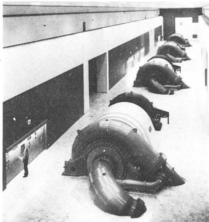
Fig. 1 Underground machine hall of the pumped-storage plant Grimsel II East
