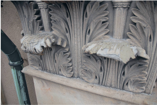
2 A Corinthian capital, bearing traces of a vain attempt around 1970 to preserve its protruding acanthus leaves by coating them with fiberglass reinforced plastics (Photo Mikael Traung).
