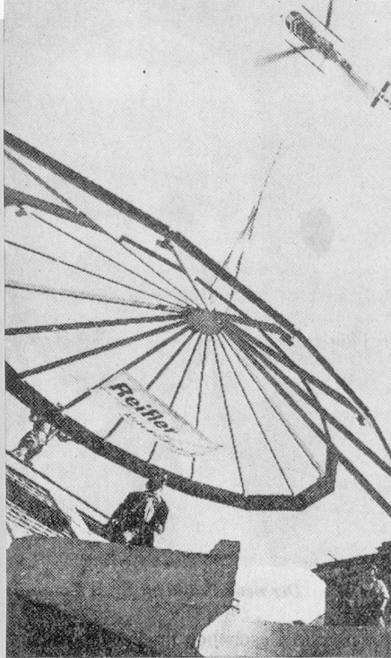
In a spectacular move, a glass dome was placed by helicopter on the top of the building housing Orell Füssli's mammoth book store.
