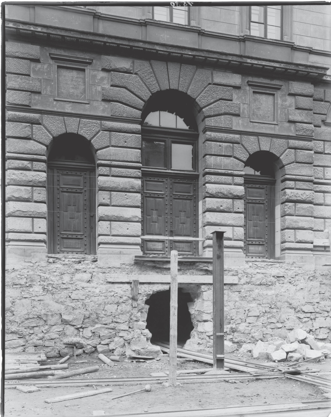
11 Gottfried Semper, Polytechnikum, Zurich; photograph of the fundamentals of the east facade during renovation, ca. 1920; Bequest of Gustav Gull, gta Archives, ETH Zurich.
