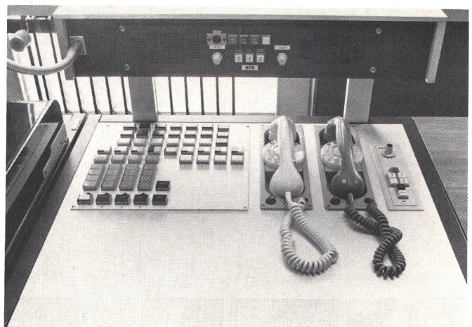
Fig. 6 View of the telephone console
