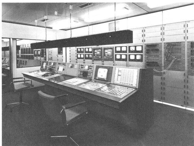
Fig. 2 Centre de commutation image – Schaltraum Video
