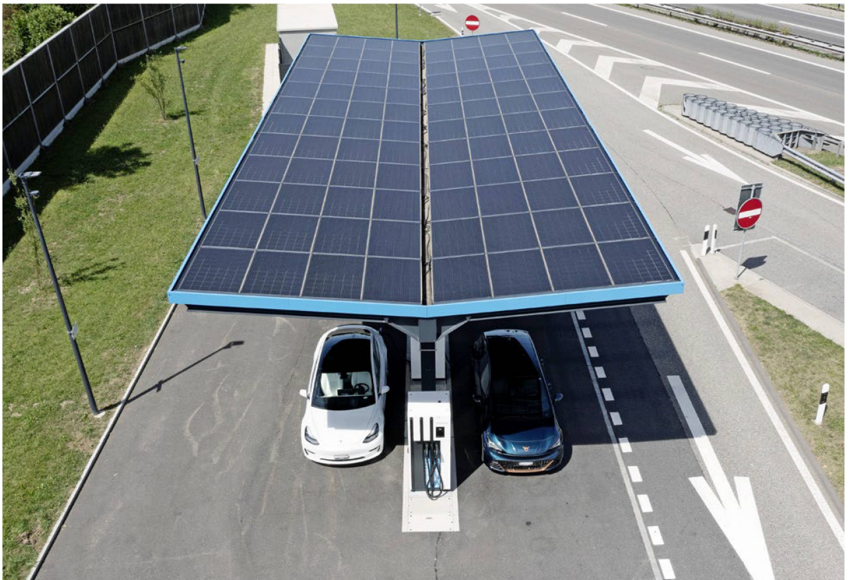
Increased electromobility means greater electricity consumption. This begs the question: how environmentally friendly are charging stations? The one pictured here near Oftringen (canton of Aargau) has a solar panel roof. Photo: Keystone
