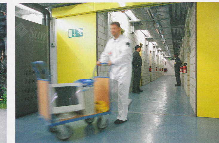
In the vaults of Swiss Data Safe
