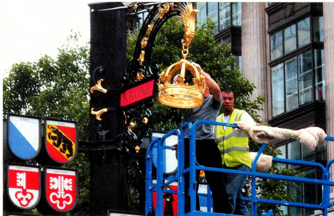
Going up: The refurbished crown is hoisted into its new position in Swiss Court
