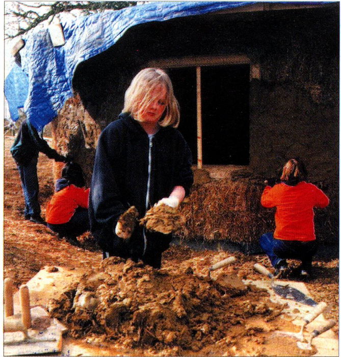
Students at work constructing a mud-and-straw building on the Pestalozzi estate in Sussex – helping them to have a greater understanding of sustainable development possibilities
