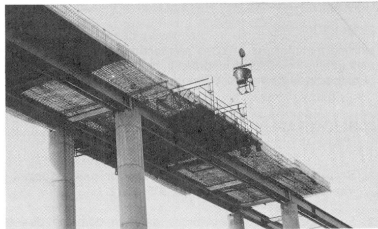
Figure 9: The bridge over the River Rance; concreting the top slab (photo G. Forquet)
