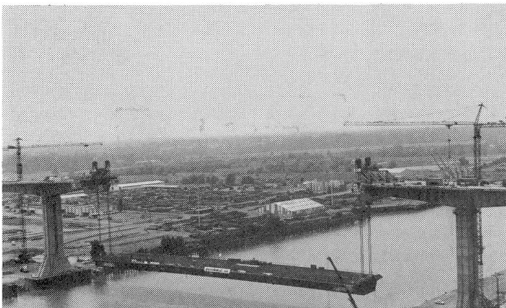
Figure 7: The Cheviré Bridge: the steel isostatic span is now lifted from the two concrete cantilevers (photo G. Forquet)
