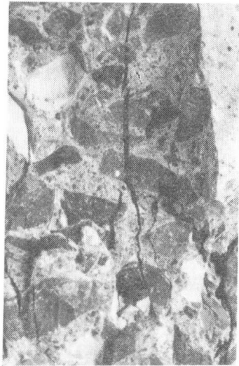
F Path of cracks
