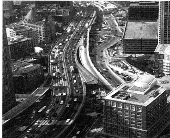
View 2 Looking along the I-93 alignment north. View shows new temporary ramp and construction below existing artery.
