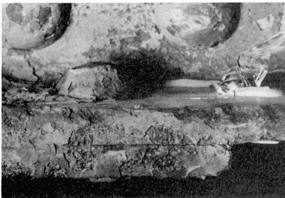
Fig. 6 Cracked angle in tension flange
