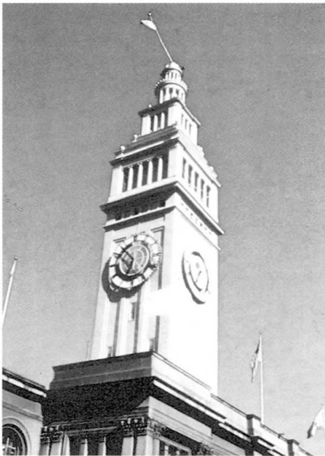
Figure 2. Photograph of Ferry Building tower after Loma Prieta earthquake with bent flagpole.
