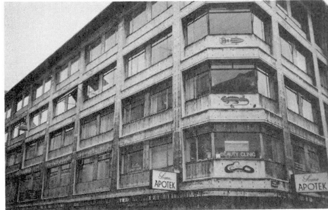
Figur 4: Miscoloured facade due to dirt and soot
