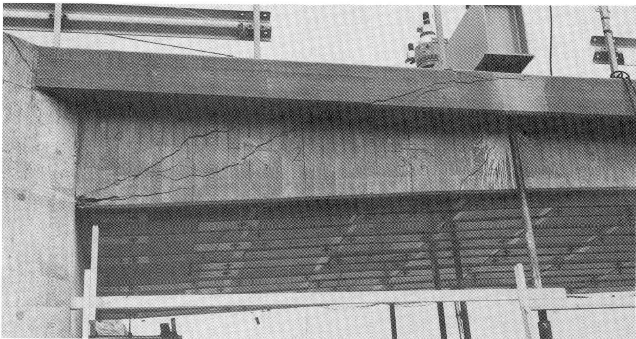
Fig. 6 Shear failure in the non-prestressed bridge
