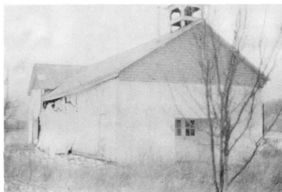
Fig. 4 Wall failure resulting from high moisture content
