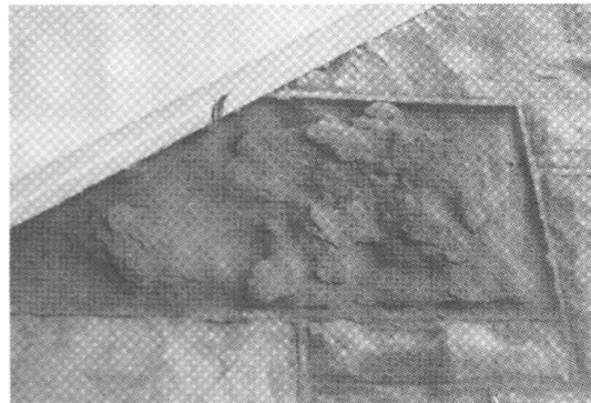
Fig. 1 Stone deterioration at repointed joint
