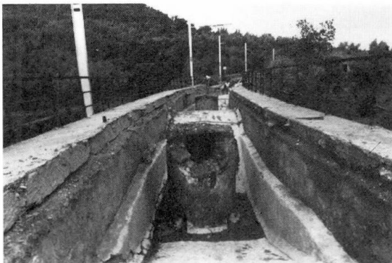
Fig. 25 The lesion in the masonry structures of the bridge.
