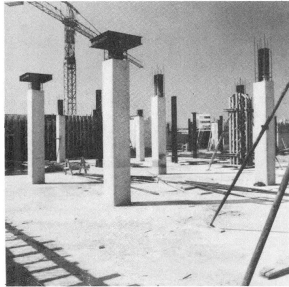
Fig. 6 Composite columns with encased hot rolled H-profiles and steel shear heads: Office building LE FOYER, Luxembourg, 1982
