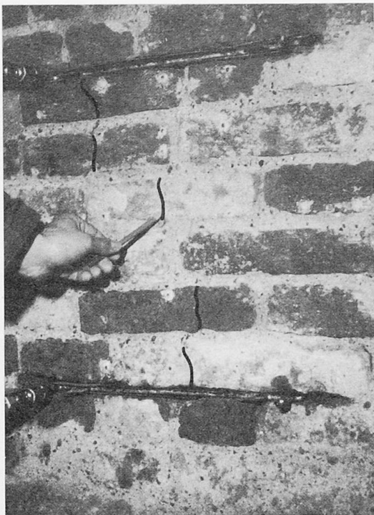
Fig. 12 Photo showing the appearance of first cracks.
