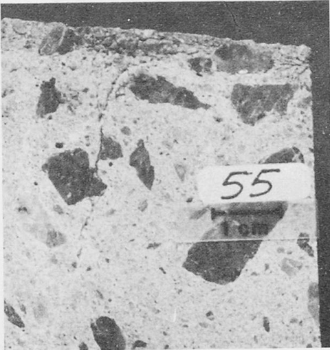
Fig. 1. Sawn cut of a concrete core with internal crack and low stone content.
