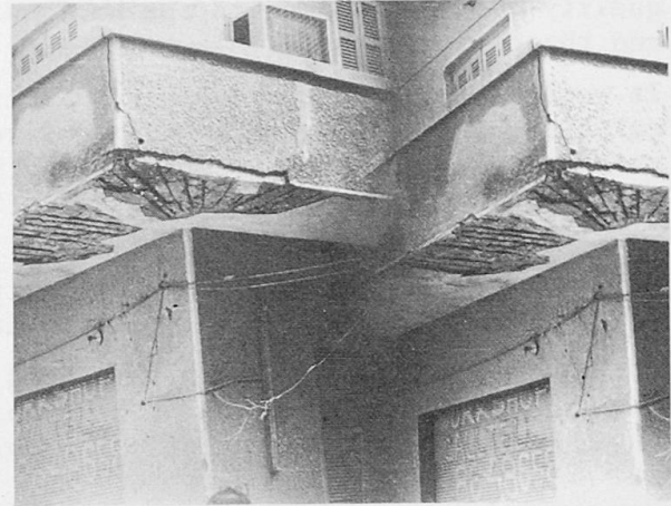
Fig. 6 Structure 2 showing concrete spalling due to rebar corrosion
