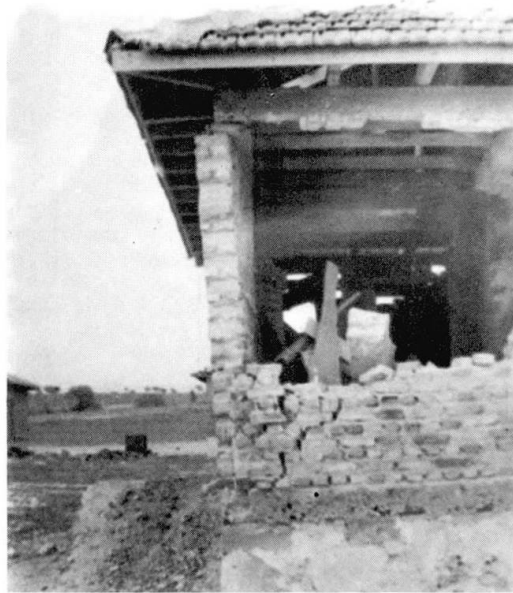
Figure-3 Corner Damage due to Earthquake
