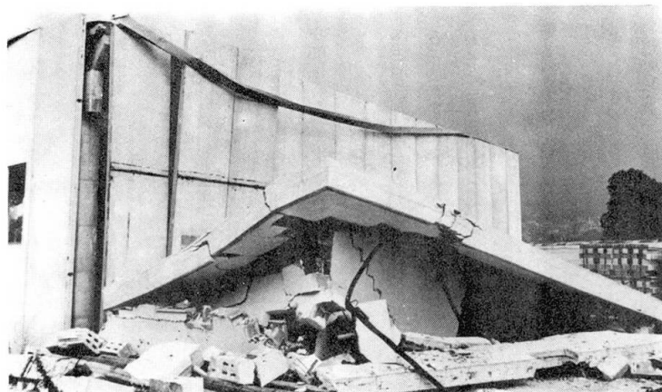
Figure 4: (after September 15th): Prefabricated shed with collapsed annex. The renewed earthquake load caused damage of the supporting framework of the shed at the fixing points of the columns and rests of the bars. The façade slabs of the side wall were severely caved in by the renewed impact: the annex itself collapsed. The increased displacement, as compared with the first earthquake, can be traced back to the reduced structural rigidity due to the destruction of one of the concrete block walls.
