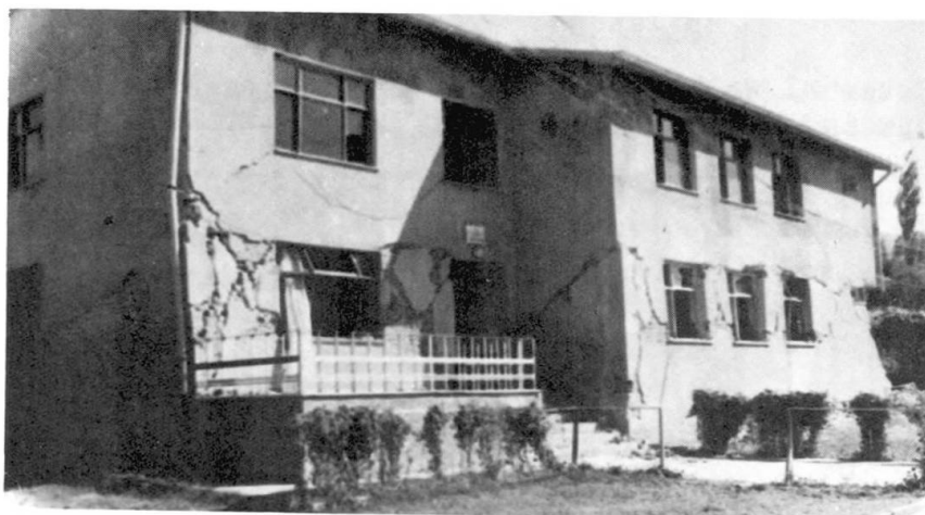
Figure-6 Typical Failure of Brick Masonry
