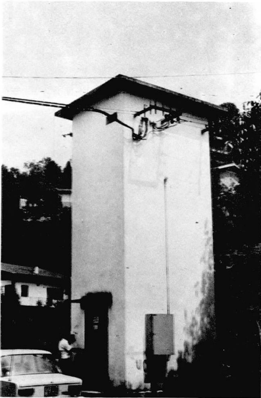
Fig 2. Distribution cabin at Bilerio.
