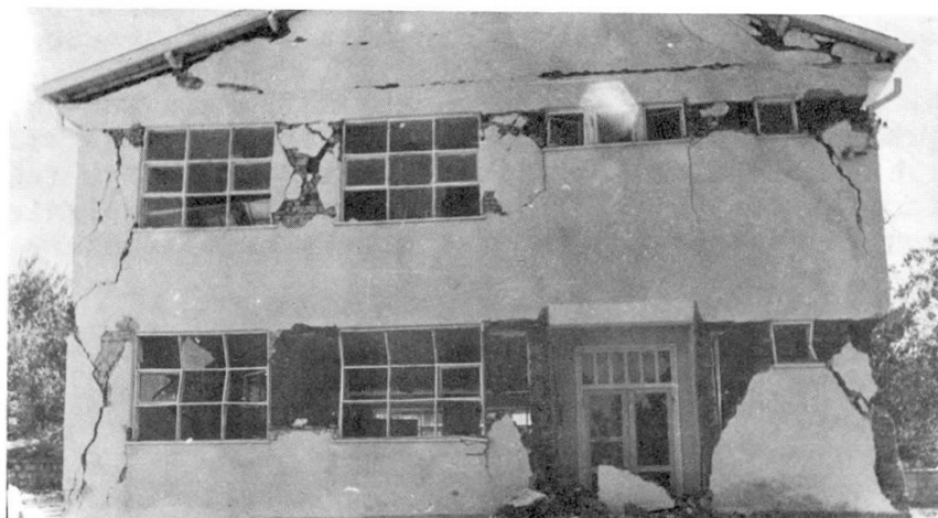
Figure-5 Typical Failure of Brick Masonry
