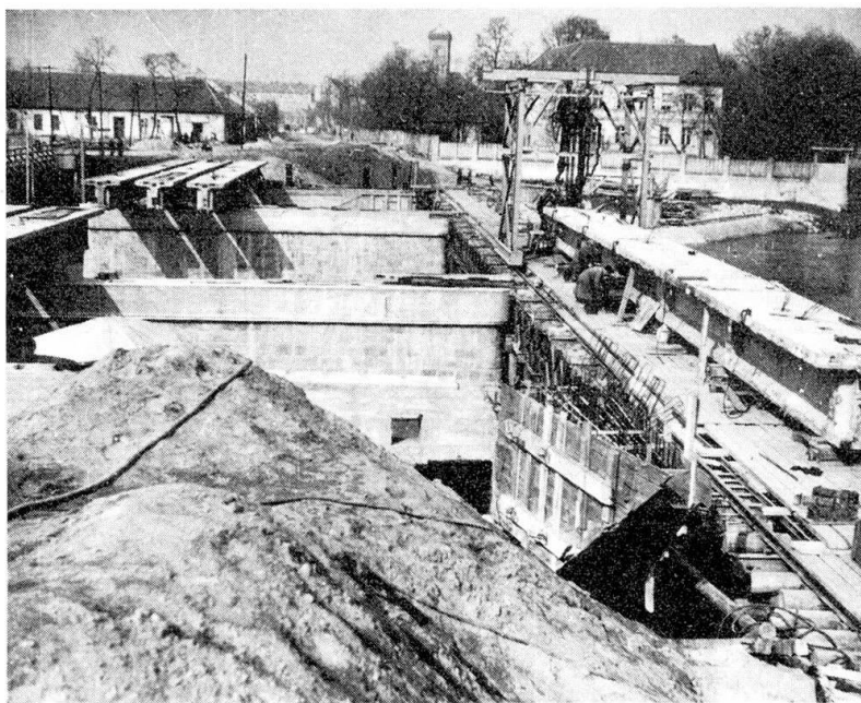
Fig.No.8.:The highway bridge " NZ " with continuous precast prestressed concrete girders during construction.
