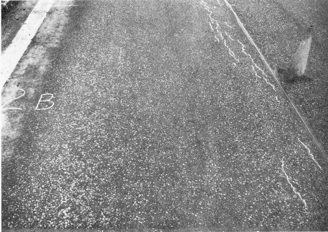
FIG. 6 CRACKING IN ROLLED ASPHALT ON FILLED RUBBER BITUMEN, NOVEMBER, 1967
