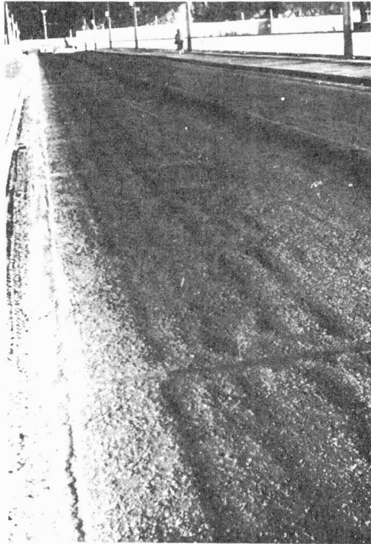
Figure 6: Rutting (transverse waving)
