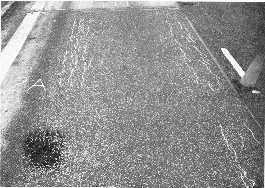
FIG. 4 CRACKING ON ROLLED ASPHALT OVER GRITTED EPOXY RESIN, NOVEMBER, 1967
