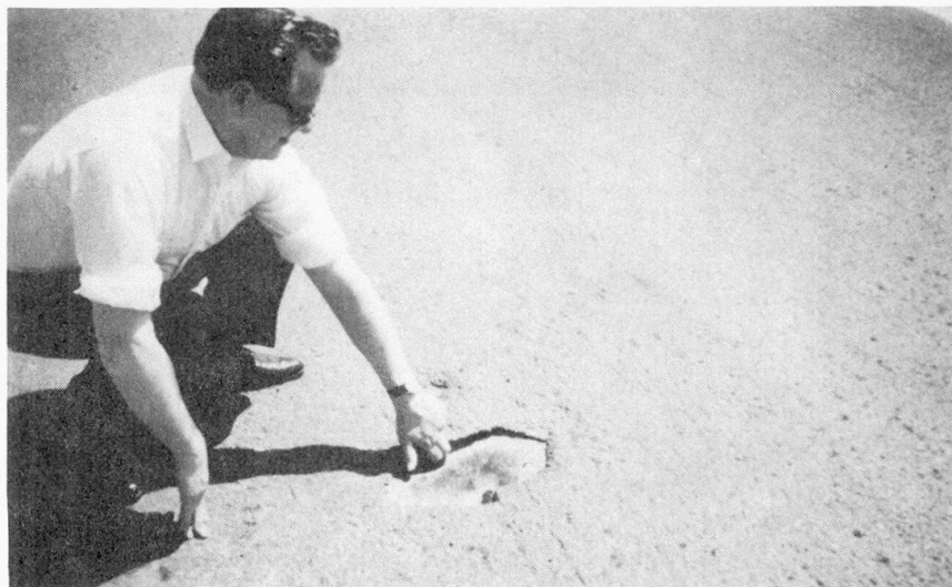
FIGURE 5. BREAKOUT OF WEARING COURSE OVER SPLICE PLATE ON CONCORDIA BRIDGE AFTER TWO YEARS OF SERVICE
