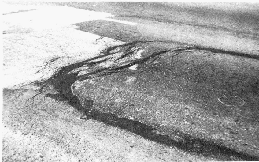
FIGURE 3. MODE OF FAILURE DUE TO DEBONDING OF THE AC PAVEMENT ON THE ULATIS CREEK BRIDGE AFTER ONLY A FEW MONTHS IN SERVICE
