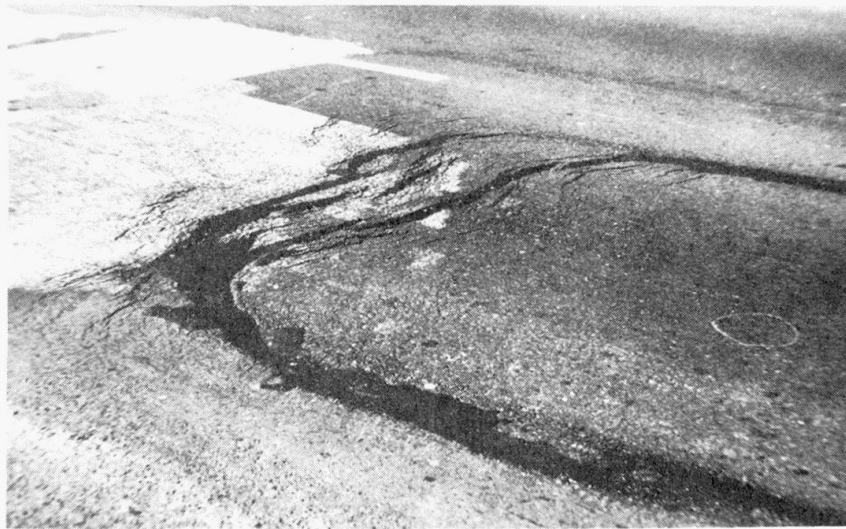
FIGURE 3. MODE OF FAILURE DUE TO DEBONDING OF THE AC PAVEMENT ON THE ULATIS CREEK BRIDGE AFTER ONLY A FEW MONTHS IN SERVICE
