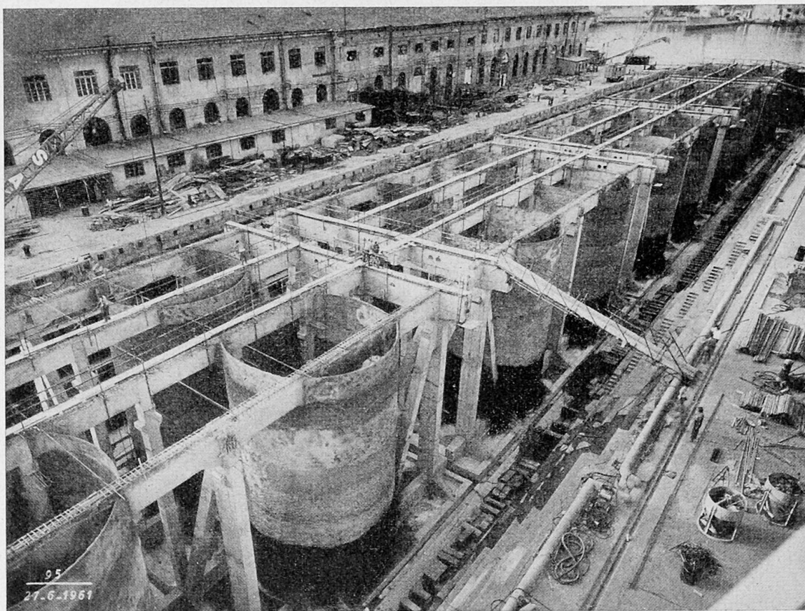
Fig. 13 - Edisonvolta thermal power plant, La Spezia. In-situ prefabrication of the fuel discharging wharf (Impresa SALCI).
