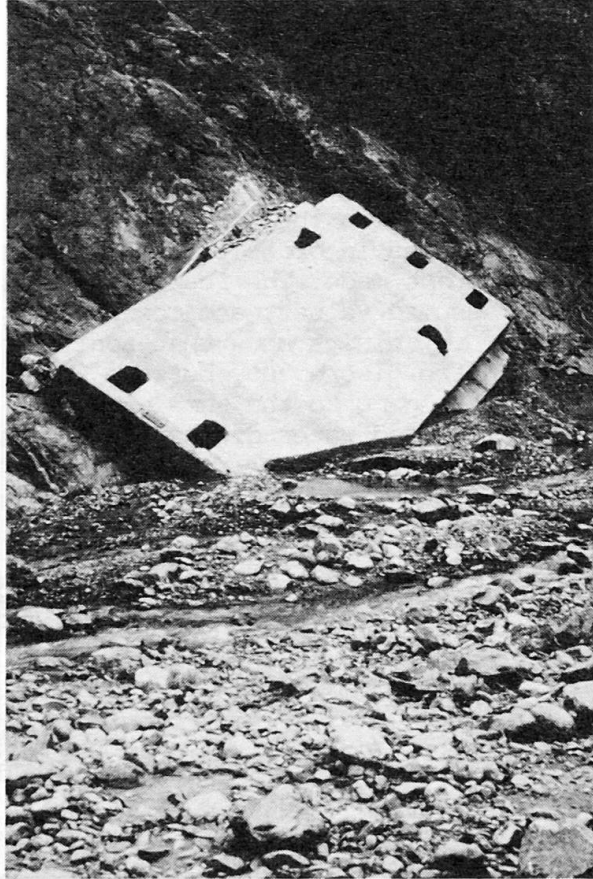
FIG. 2 200 Ton Bridge slab after the flash flood.
