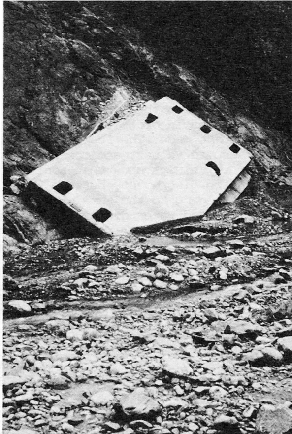
FIG. 2 200 Ton Bridge slab after the flash flood.
