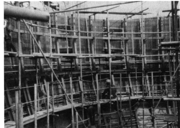
Fig. 3 View of the formwork; note the block-out forms for the horizontal post-tensioning
