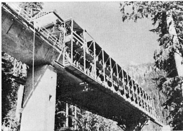
Fig. 1 Movable truss scaffold moves from pier to pier across the valley of Denny Creek, leaving behind the bottom and sides of post-tensioned box girder that will support the forms for casting the top and deck of the bridge superstructure.
