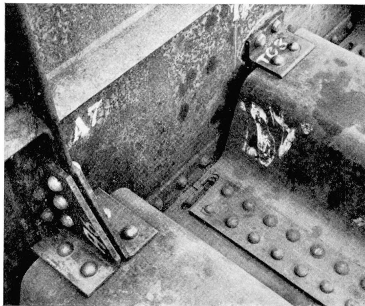
Fig. 13. Transverse pressed steel troughing connected to a main girder by cleats at the top and by plug-welds at the bottom
